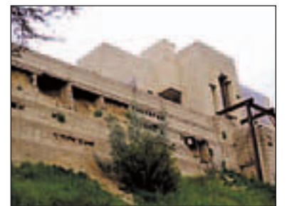
Severe storms have weakened the Ennis-Brown House, a 1924 Frank Lloyd Wright building in Los Angeles.
